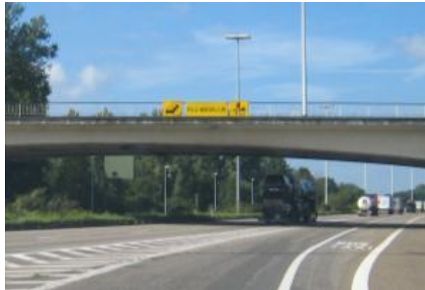
Fixed signs warning about queue likeliness (here 4600m before the work zone)
